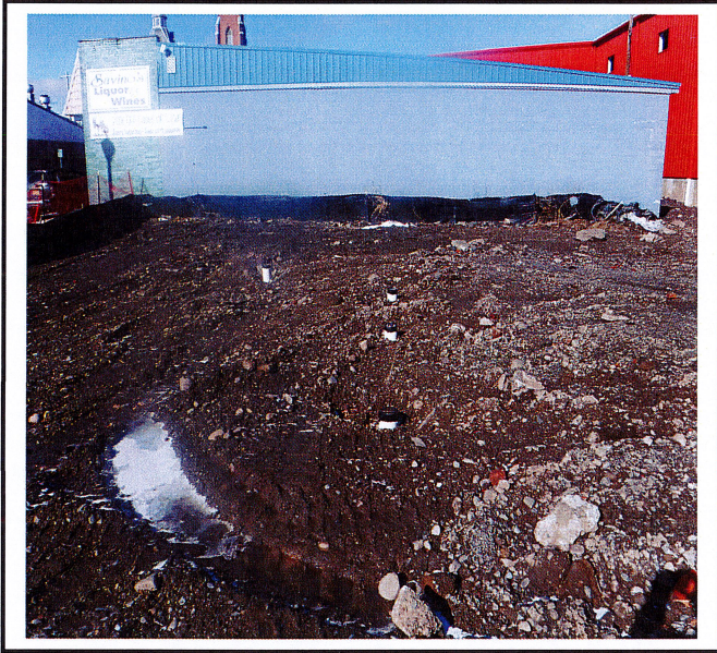
Underground stormwater system was installed. Does not appear C&D was removed from area as SWPPP was approved.
