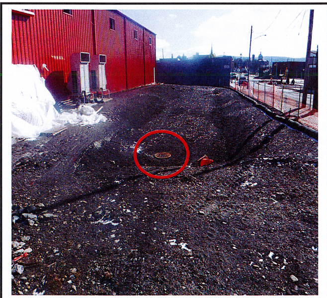
Closed lid on dry well should be an open grate so water can get into it.
