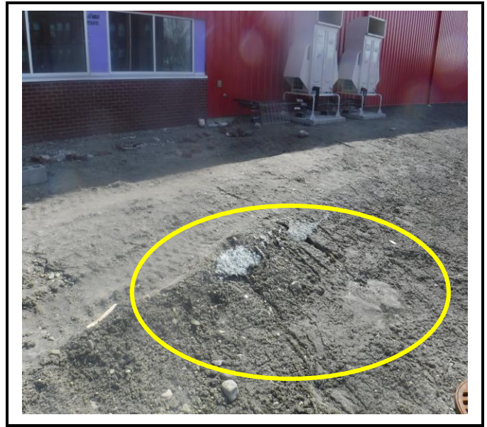
Erosion has started on the side slopes of the rain garden.
