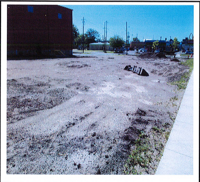
Future green area next to building and above the underground infiltration has not been stabilized.
