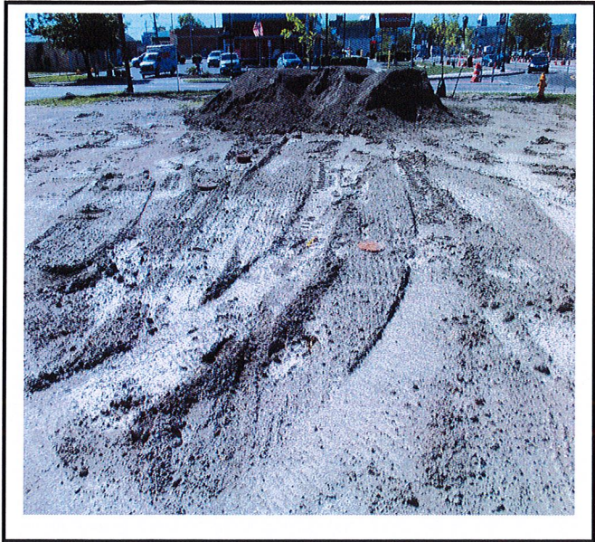
Topsoil was stockpiled on top of underground infiltration and one of the observation ports has been hit by equipment.
