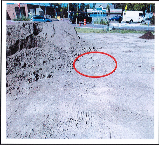
Topsoil was stockpiled on top of underground infiltration and one of the observation ports has been hit by equipment.
