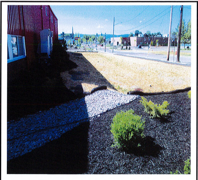
Rain Garden- repairs have been made to eroded areas but landscaping is not completed.
