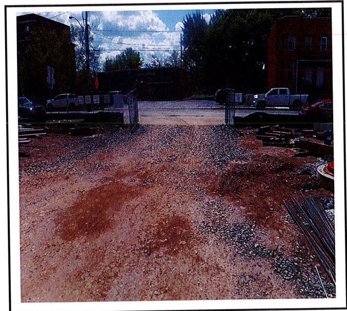
2 nd Construction entrance requires maintenance.
