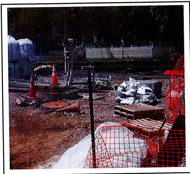
Water quality unit that is part of the underground stormwater facility is surrounded by mortar mixing materials. SEE INSPECTION NOTES
