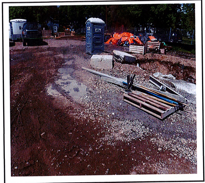
Concrete wash water all over the area surrounding the concrete washout.
