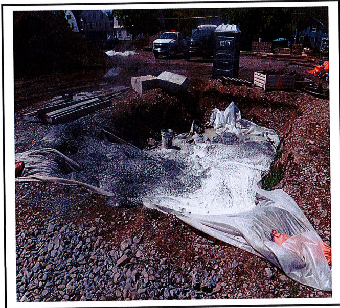
Concrete washout requires immediate maintenance.
