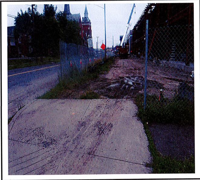
Traffic moving through area without construction entrance.
