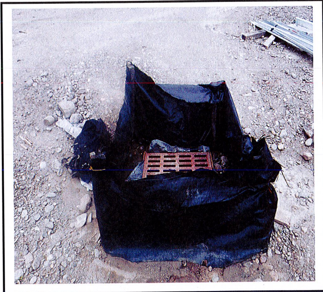
Wooden top rail not installed.
