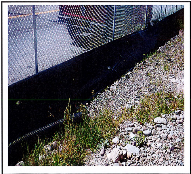
Silt fence along Clinton Street has holes and is in need of repair.
