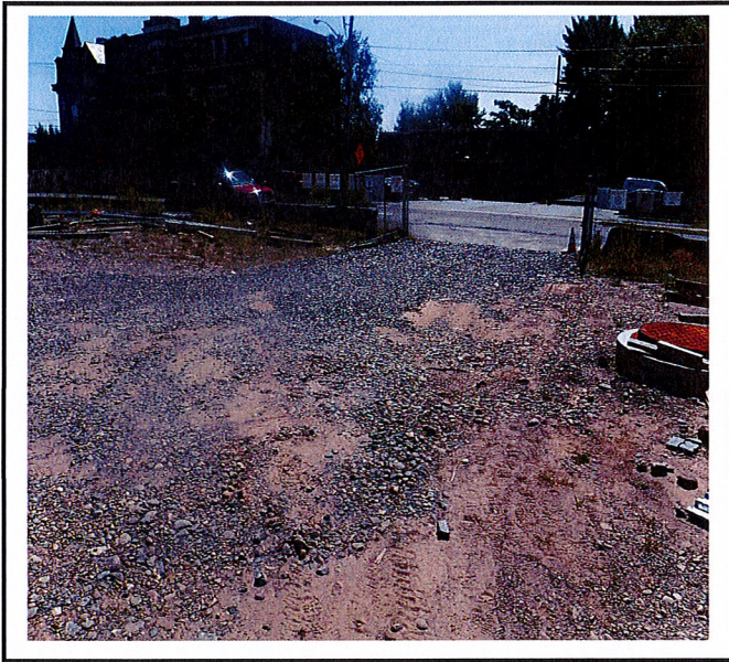
Construction entrance in fair condition although sediment from project site is tracked up Clinton Street and W. Fourth Street.
