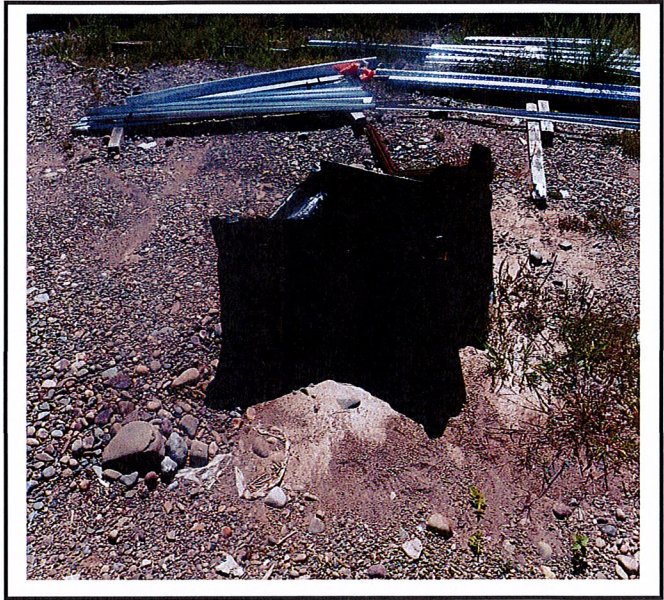
Drop inlet protection around CB-2 remains installed incorrectly.
