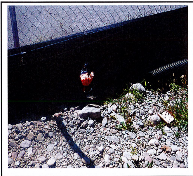
Silt fence along Clinton Street has holes and is in need of repair.
