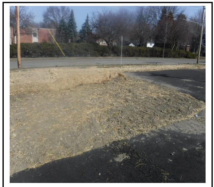
Soil is not stabilized or protected from erosion.
