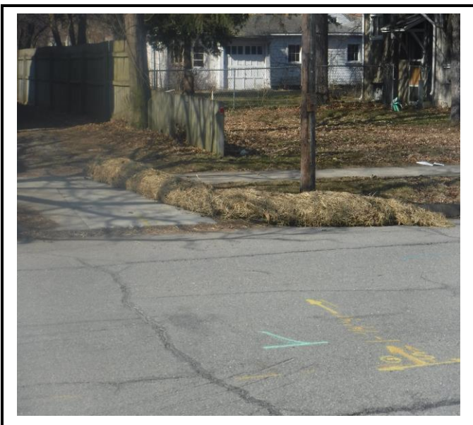
Rolled erosion control blanket was not secured properly. This photo shows a whole section blown across the street into a neighbors yard.
