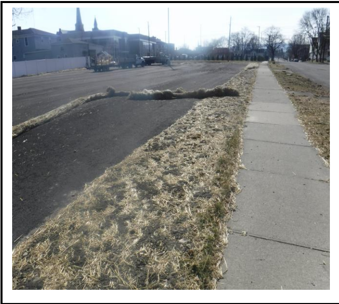
Rolled erosion control blanket has blown off the area that it was supposed to be protecting.
