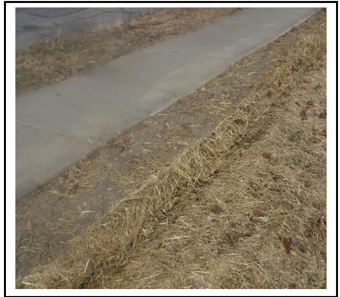
Rolled erosion control blanket was not secured properly to the soil and now has blown back. Soil is exposed and unprotected.
