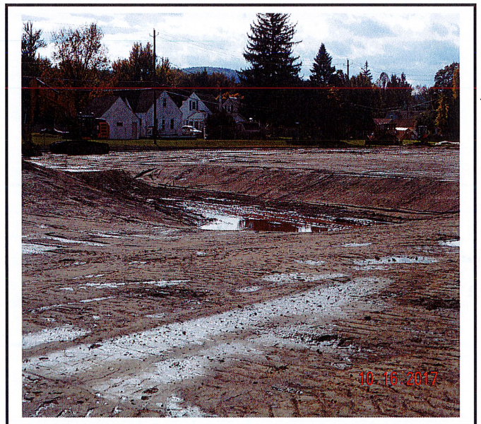
Forebay has been cut in for use as a sediment trap. It has not been brought down to final grade.
