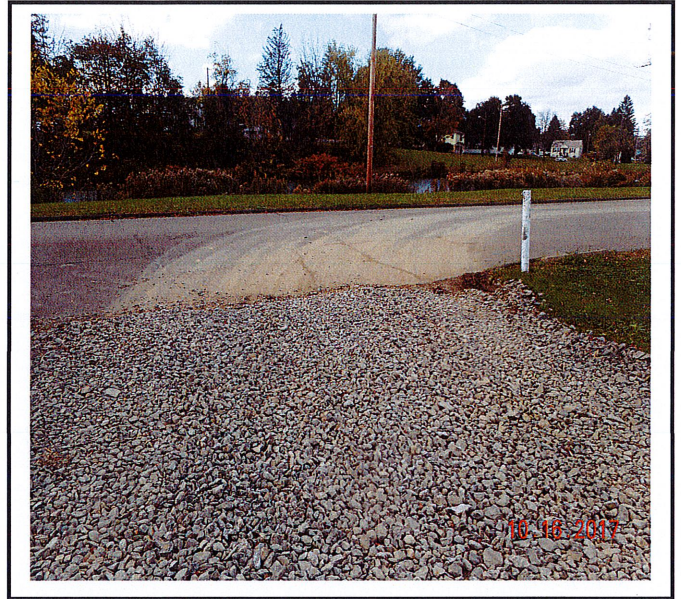
Construction entrance-there is slight tracking out onto the road.
