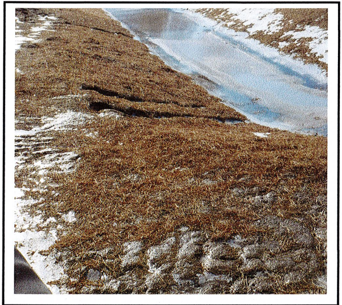
Erosion on the side slope of western most forebay (back of property).
