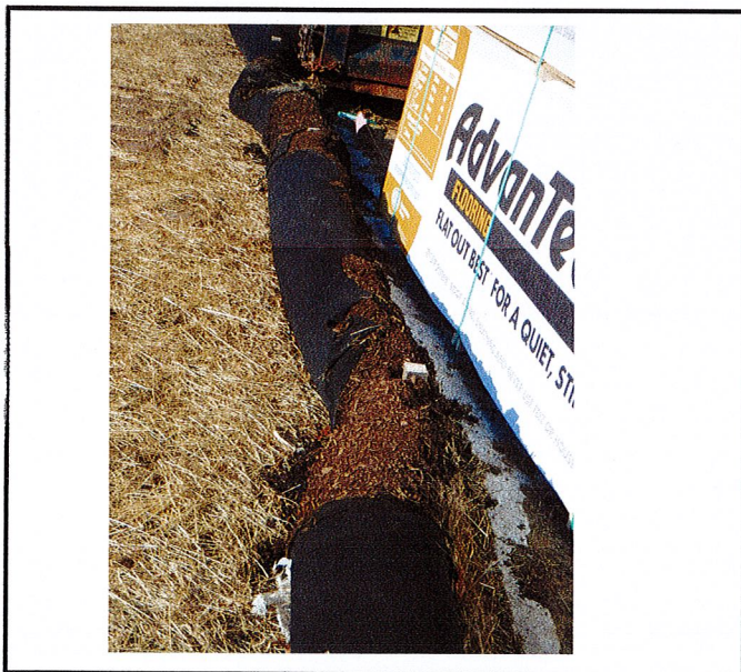
Compost sock ripped apart. This will not function once thawing occurs.
