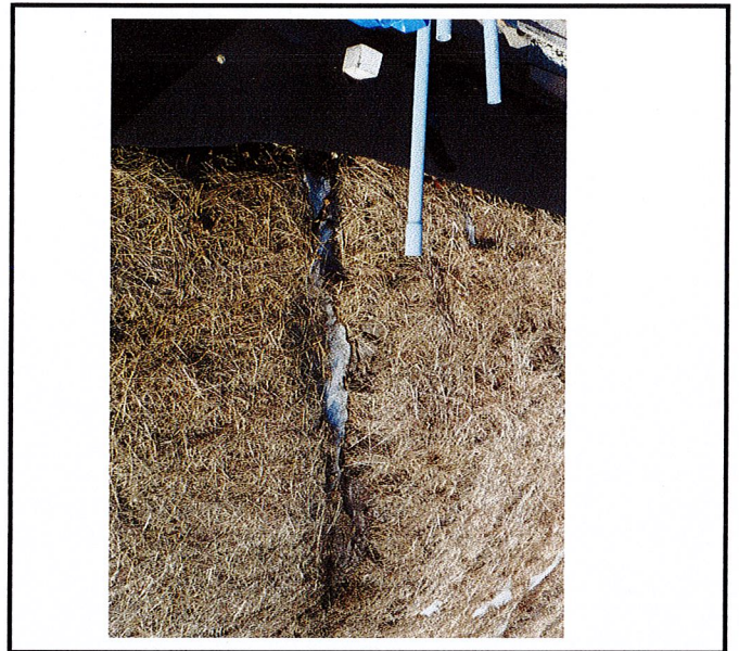
Water is getting under the compost sock and causing erosion on the side slope of the infiltration basin.
