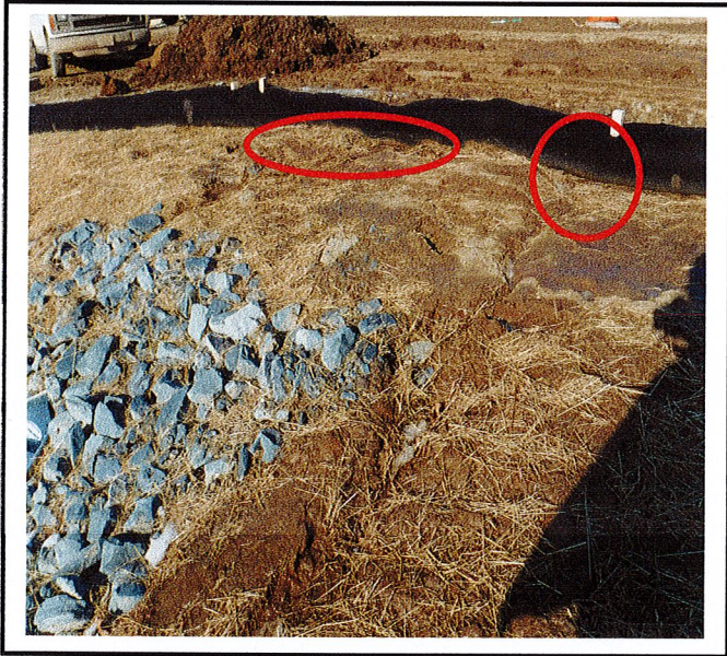
Water is getting under the compost sock and causing erosion on the side slope of the infiltration basin.
