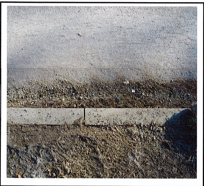
Contractor swept Maple Ave but failed to sweep up material to prevent it from getting into storm drain.
