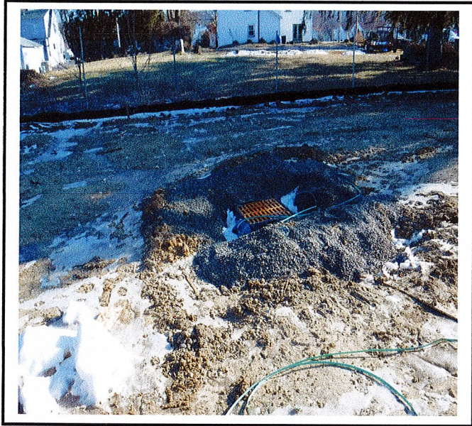
Outer stone drop inlet protection needs repair.
