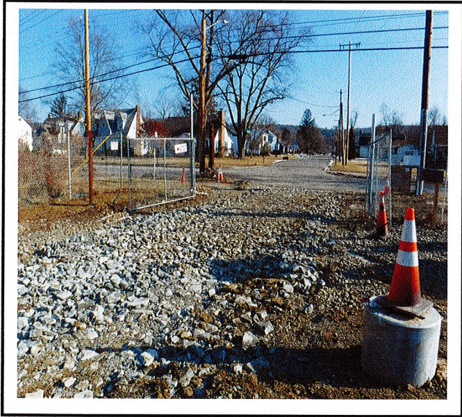
Construction entrance is worn out and mud is being tracked onto Maple Ave.
