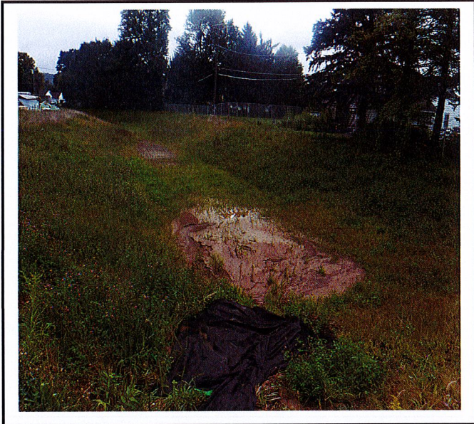
Sediment accumulated from contractor pump down and erosion into the infiltration basin.
