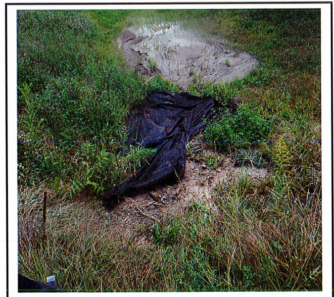
Erosion into the west end of the infiltration basin. Erosion caused by contractor pumping down west forebay into sediment bag.
