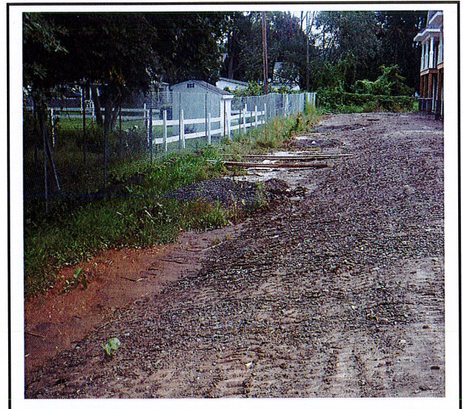
Area to the north of the building - Erosion is occurring down the side slope-stabilization and soil restoration needed.
