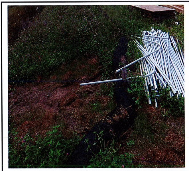
Erosion occurring into the east forebay.
