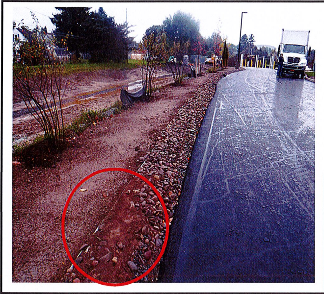
Water quality trench needs to be graded. Also, sediment has been placed on the trench.
