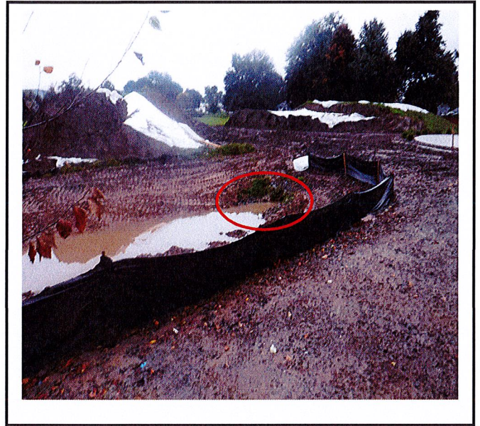
Outlet protection appears to have been removed during re-grading.
