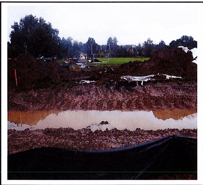
Outlet protection on roof outlet line has not been installed.
