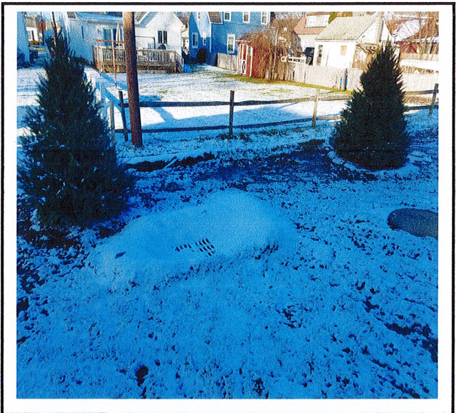
Water is standing up along edge of silt sock. This area needs to grade to the catch basin when final grading is completed.
