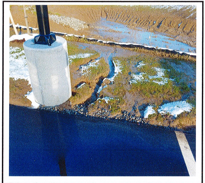
Erosion off parking lot into forebay
