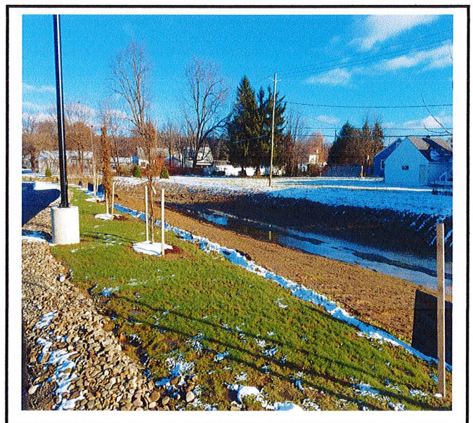
Standing water in infiltration basin.
