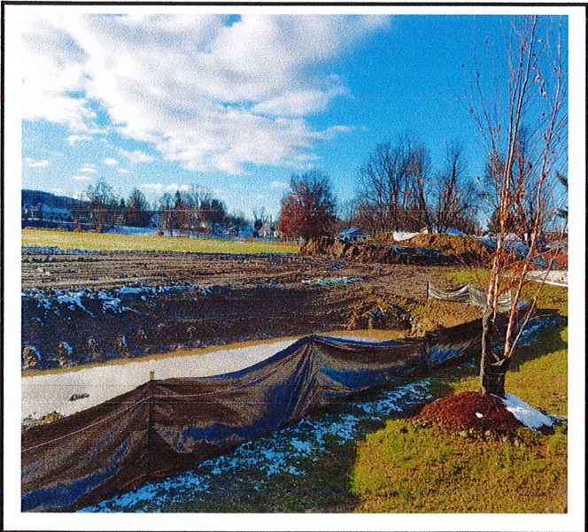
Stockpile area has not been removed or stabilized.
