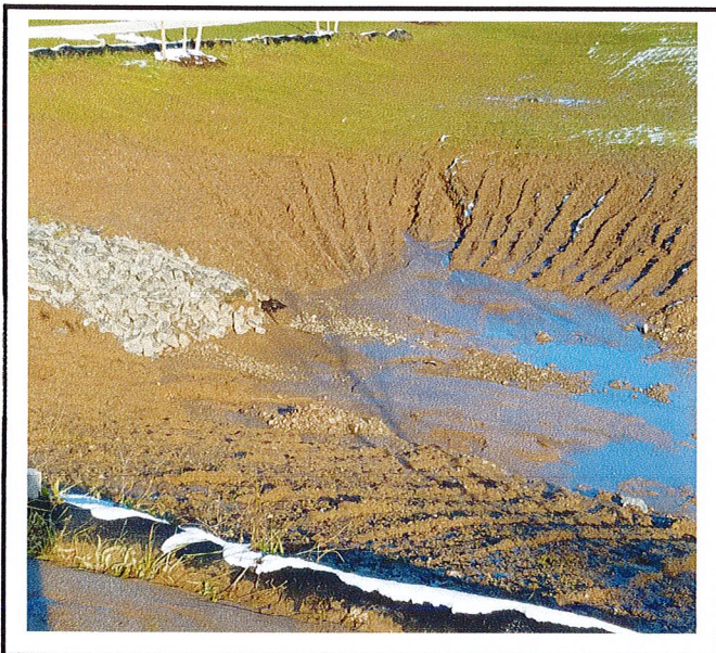
Erosion continues into forebay. Sediment is accumulating on bottom.
