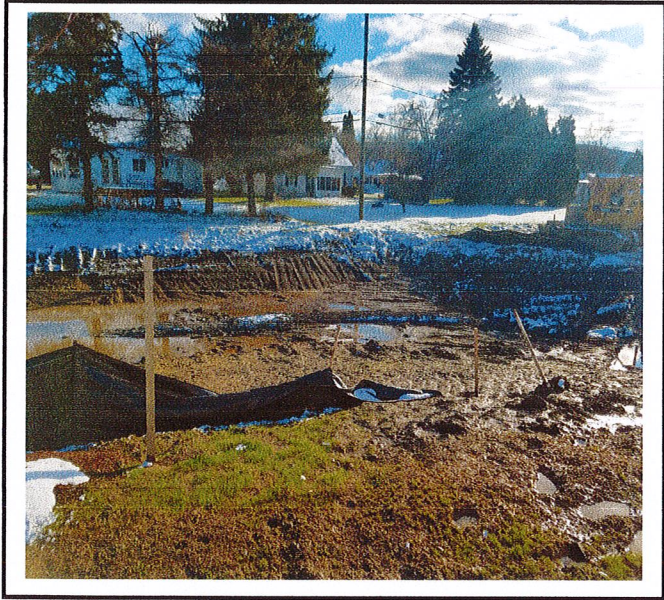
Silt fence requires repair.
