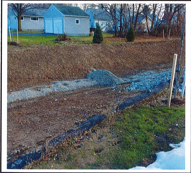
Stone berm does not appear to be installed correctly.
