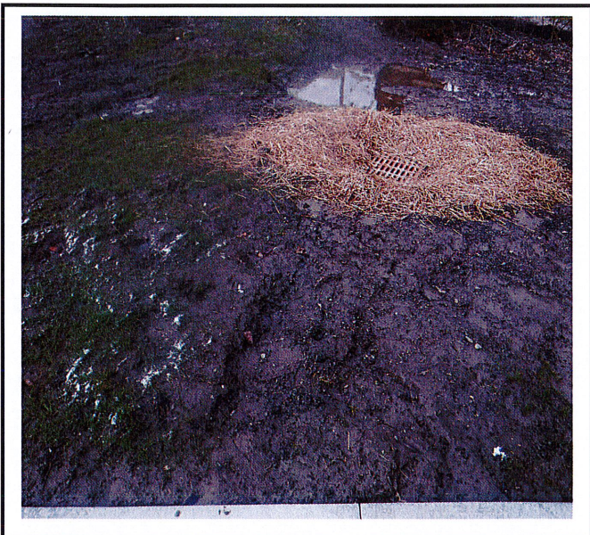
Erosion occurring off back sidewalks down to catch basin.
