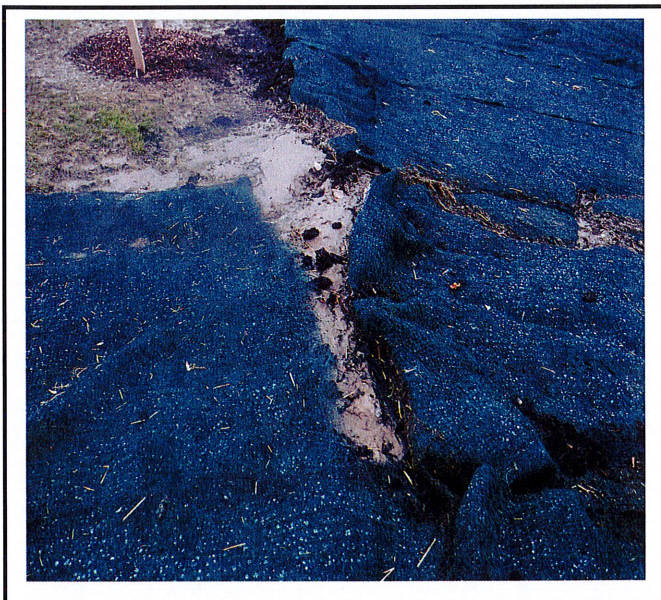
Blankets not installed correctly.
