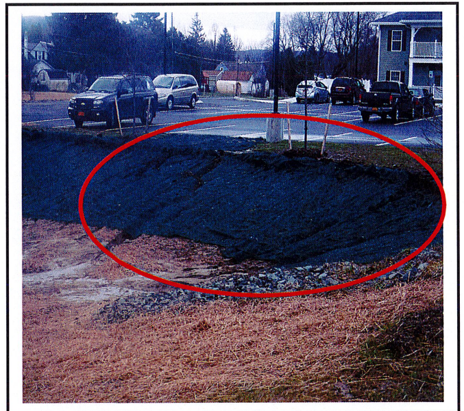
Erosion is occurring from surface runoff off from the parking lot.
