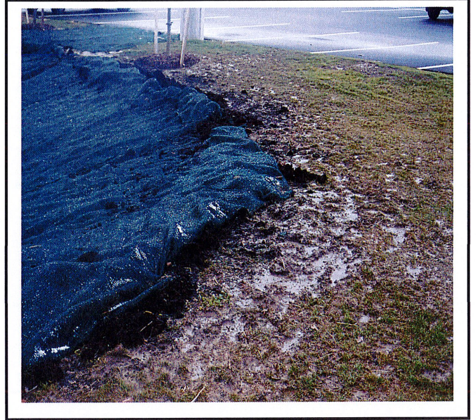
Erosion control blanket not correctly installed. It appears the compost sock was cut open and the blanket was tucked under that.
