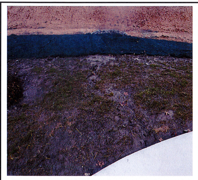
Erosion occurring off area near dumpster. This will eventually get under the blanket and cause sediment building up in basin.
