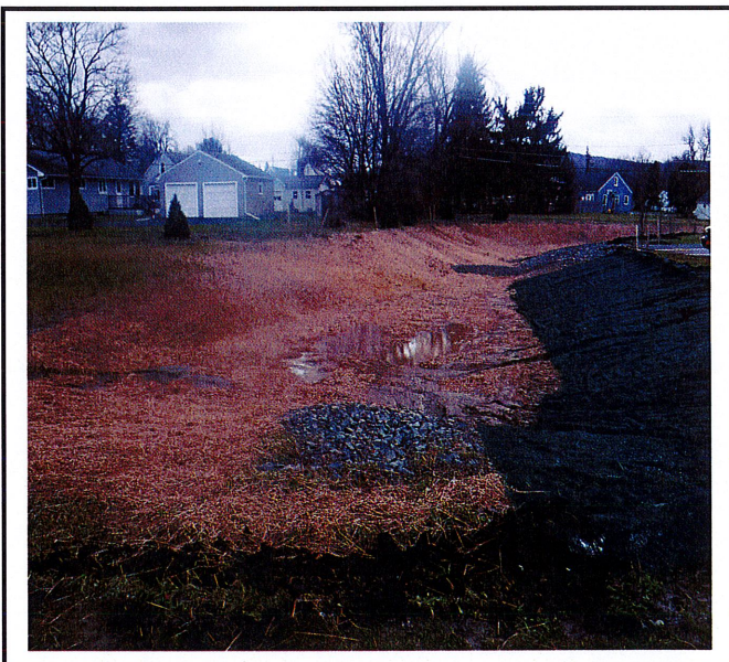
All bare soil has been covered but there is major erosion still occurring.
