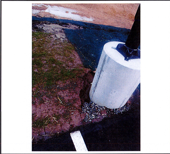
Erosion occurring from surface runoff from parking lot.
