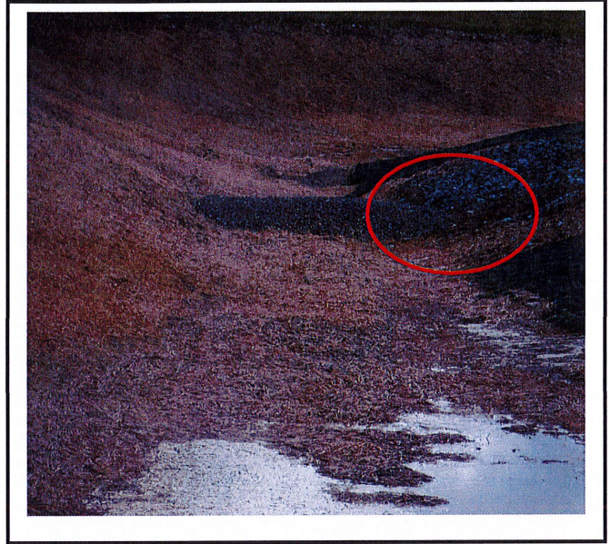
Rock berm is not installed correctly. Water can get around the berm in this section.
