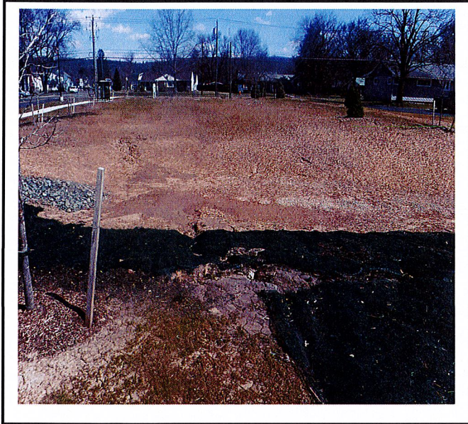
Surface runoff from parking is causing erosion down slope of stormwater basin.
