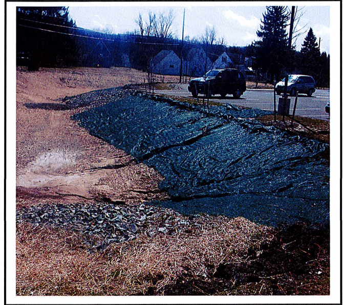
Erosion that has occurred. Check dam has not been installed correctly.
