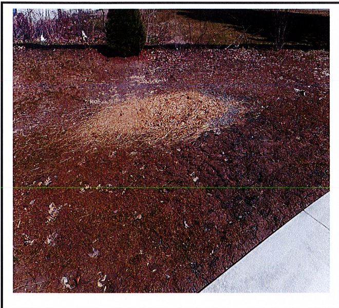
Erosion started from runoff over sidewalk to catch basin.
