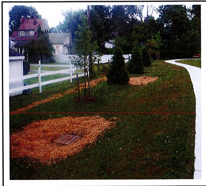
Grading around catch basins have been corrected.
