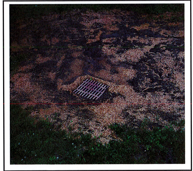
Catch basin is receiving a lot of runoff has washed seed and mulch. The straw and seed will have to be re-done.
