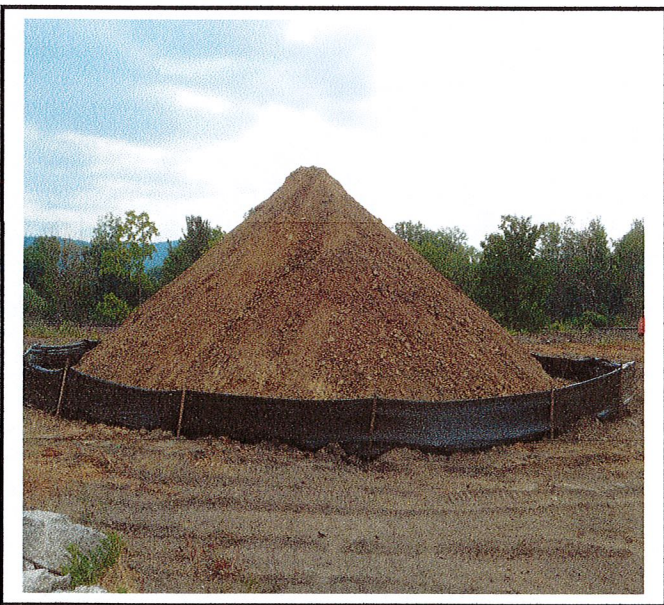
Topsoil pile needs to be temporarily stabilized.
