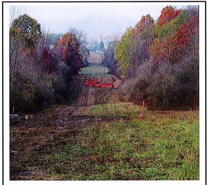
Area where working outside of LOD and soil stockpile.
