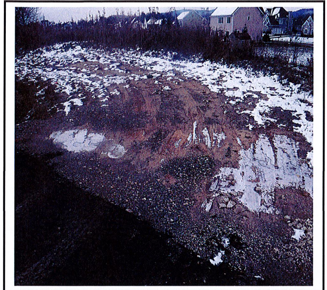
Contractor utilizing Lot #86 and there is slight sediment tracking onto road. Construction entrance will be necessary if use is continued.
