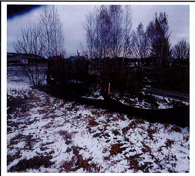
Silt fence requires maintenance in a few spots.
