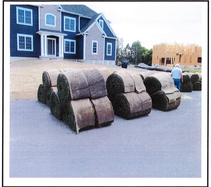
Sod delivered morning of this inspection.
