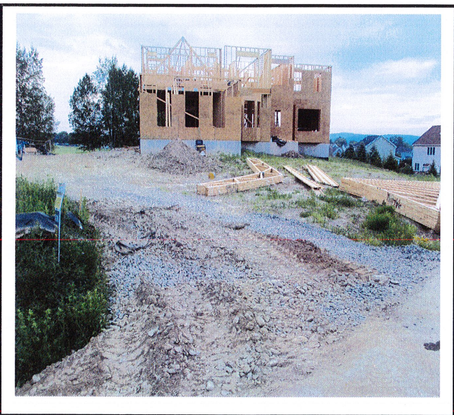
Monitor construction entrance on Lot 86. Sediment is tracking to road.
