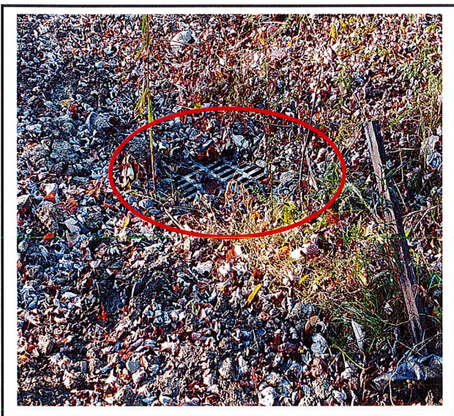
Catch basin requires protection.
