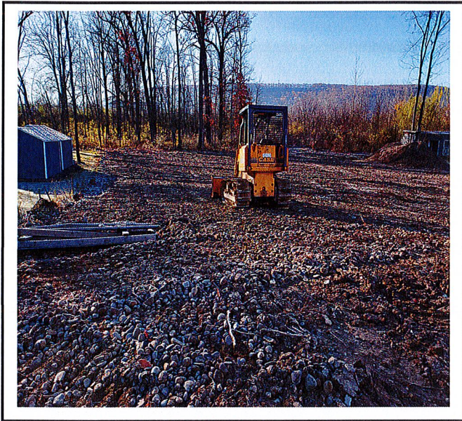
Exposed soil needs to be seeded and mulched.
