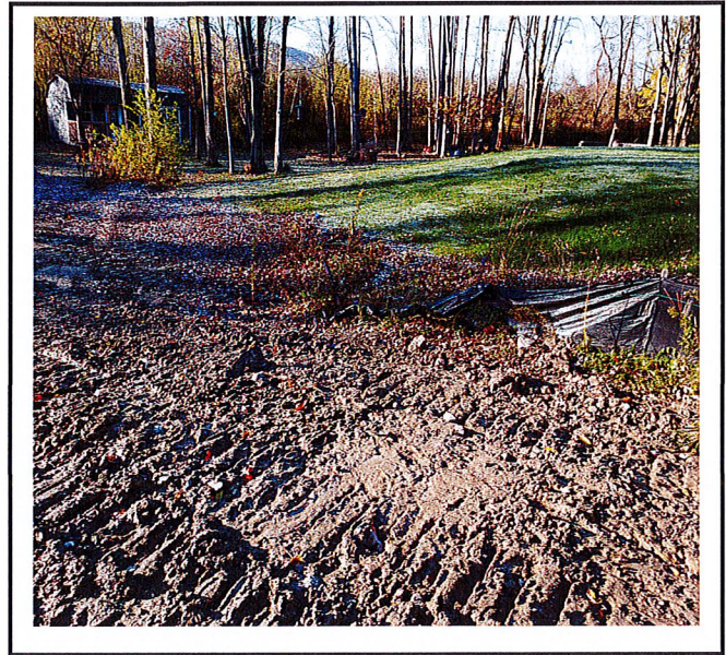
Silt fence needs to be replaced and soil needs to be stabilized.
