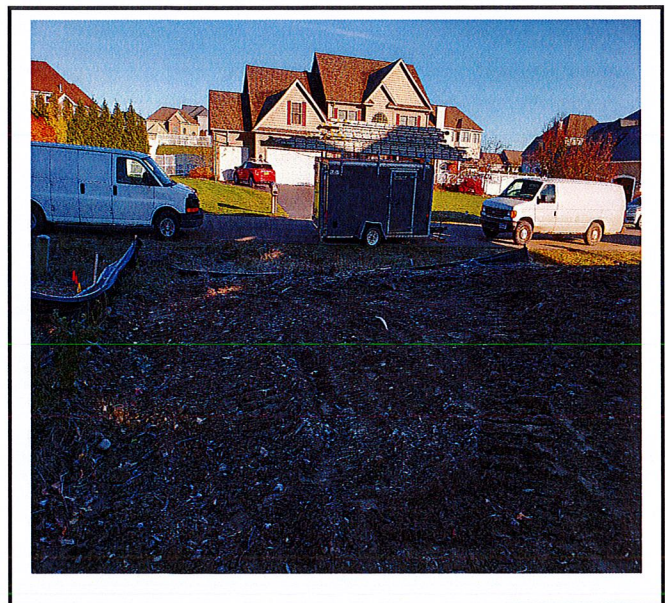
Silt fence needs to be replaced and stabilization of exposed soil in areas where contractors are not working.
