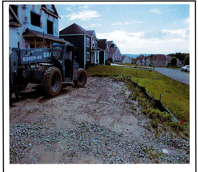
Bare soil outside of a 10' perimeter around the house needs to be temporarily stabilized. Soil is eroding and leaving the site.
