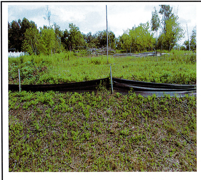
Silt fence around both lots needs to be replaced with new silt fence. Existing fence has holes and is beat up and cannot be salvaged.
