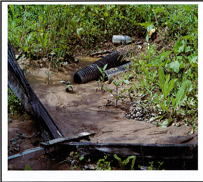
Sediment has overrun the silt fence and left the project location.
