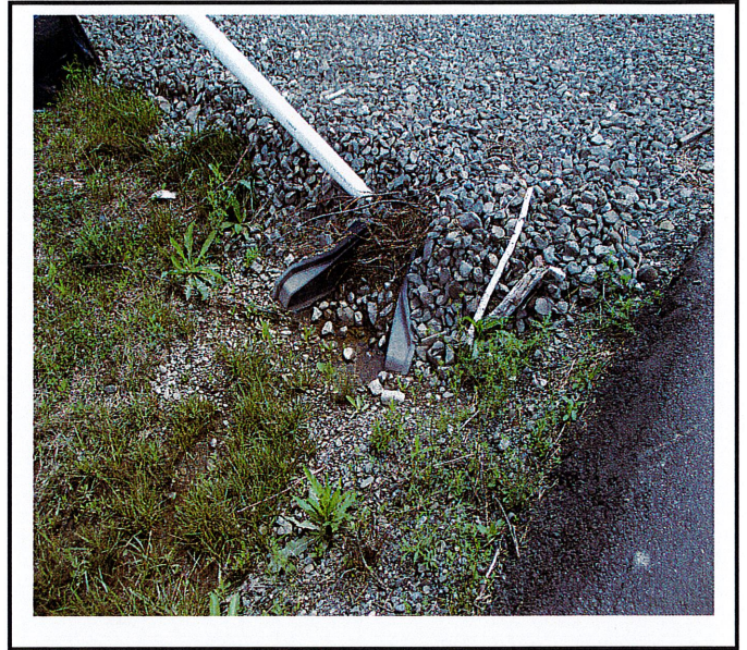
Driveway culvert pipe is blocked with stone and veg. debris. This disrupts flows from other areas of the neighborhood.
