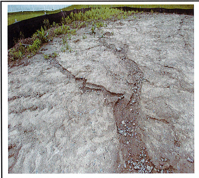
Erosion is occurring around the entire lot. Soil has not been stabilized and it is well past 14 days sitting idle.
