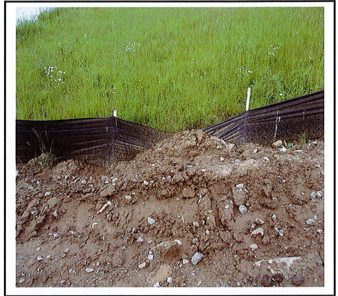
Silt fence needs to be maintained at different spots around the lot. In this photo soil is over the top of the silt fence.
