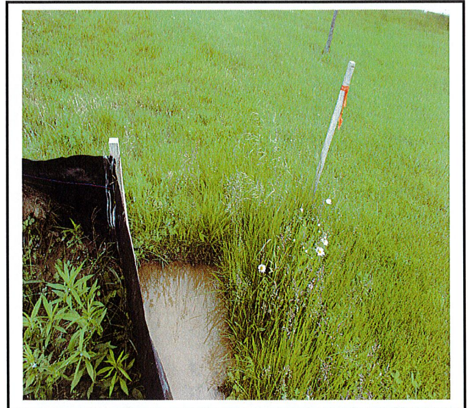
Sediment laden water is getting past silt fence.
