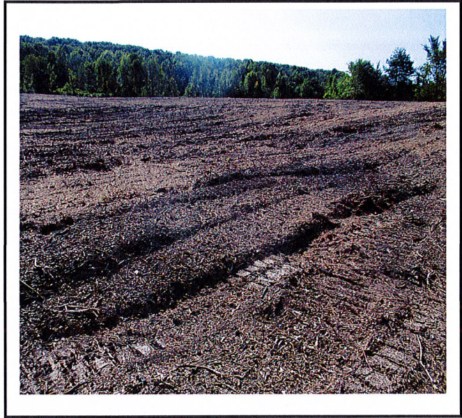
Too much soil is mixed with the wood mulch and there are many areas such as this that require further soil stabilization.
