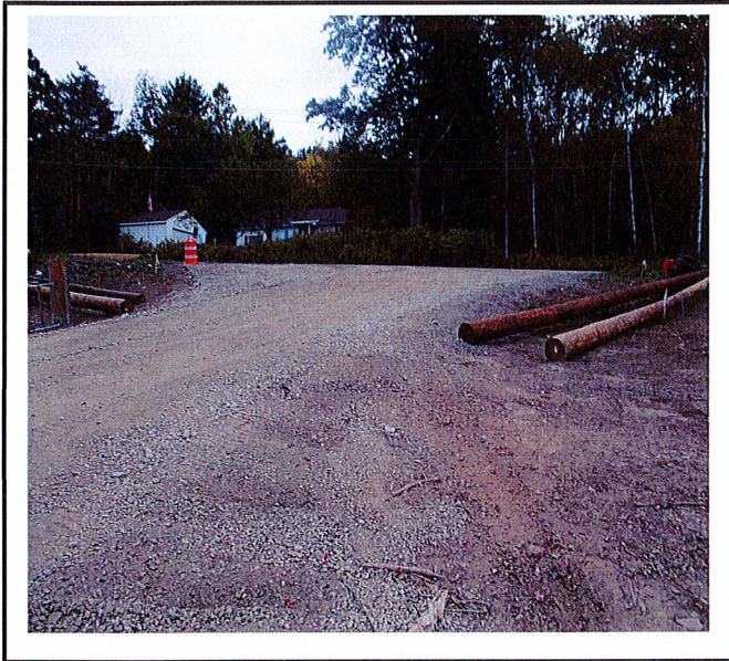
Construction entrance requires maintenance due to dust accumulation.
