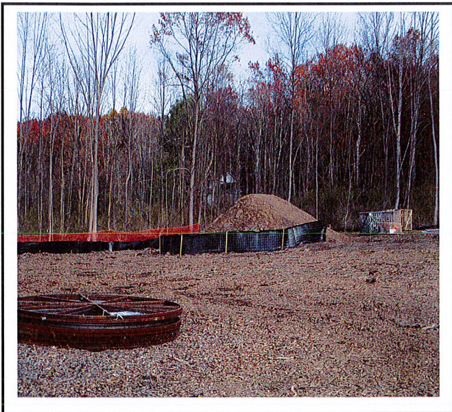
Areas overdriven during construction will require soil restoration and stabilization. Soil stockpile should be stabilized.
