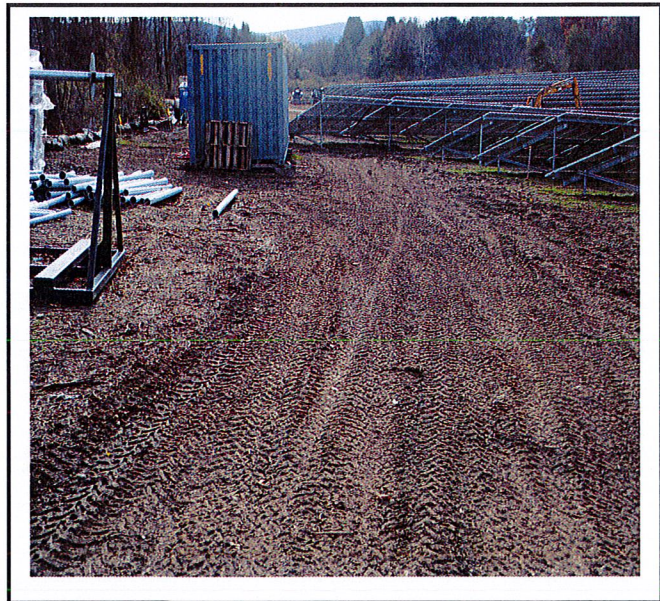
Areas overdriven during construction will require soil restoration and stabilization.
