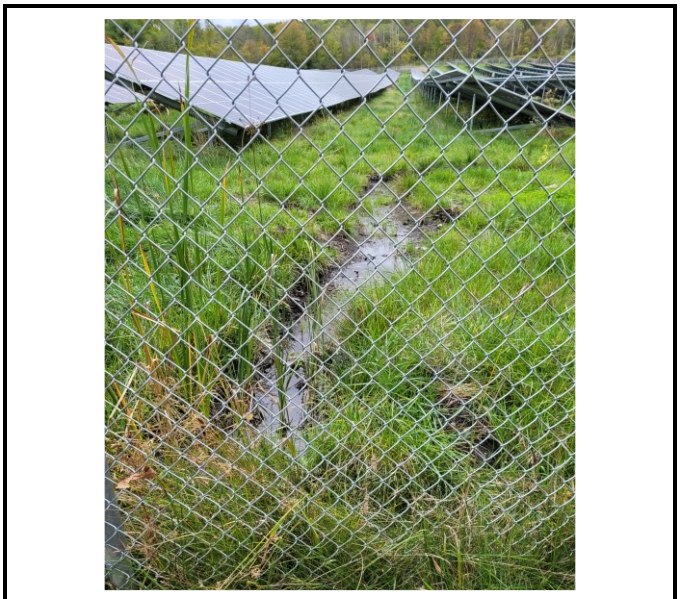
Standing water is still an issue on lower part of project inside of the fence. Now that it is raining again it is visible.
