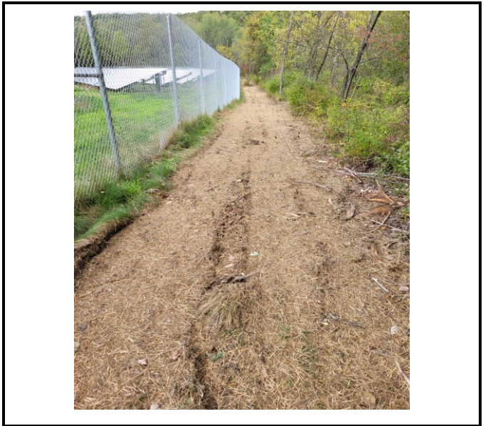
Soil restoration/decompaction and compost sock removal has been performed in some areas.
