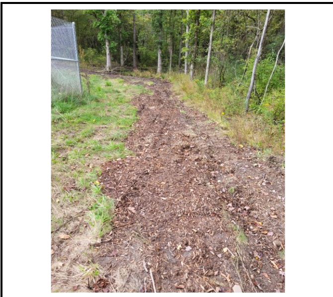
Areas where compost sock removed but not yet restored due to moisture.
