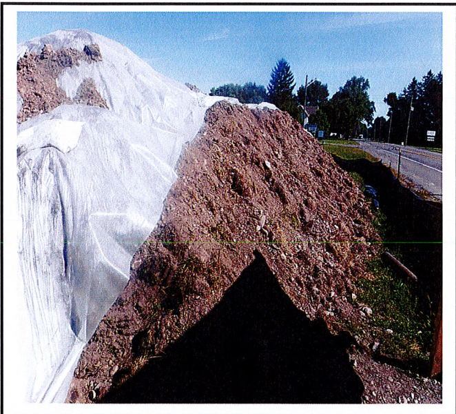
Soil stockpile is partially covered with plastic. It either has to be completely covered or temporarily stabilized.
