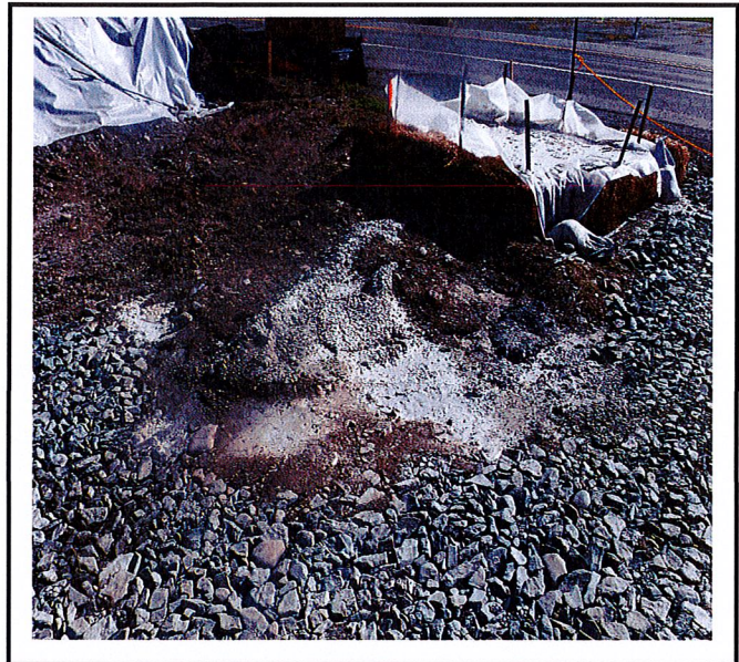
Concrete washout is 100% full and concrete has been washed onto the ground next to washout pit.
