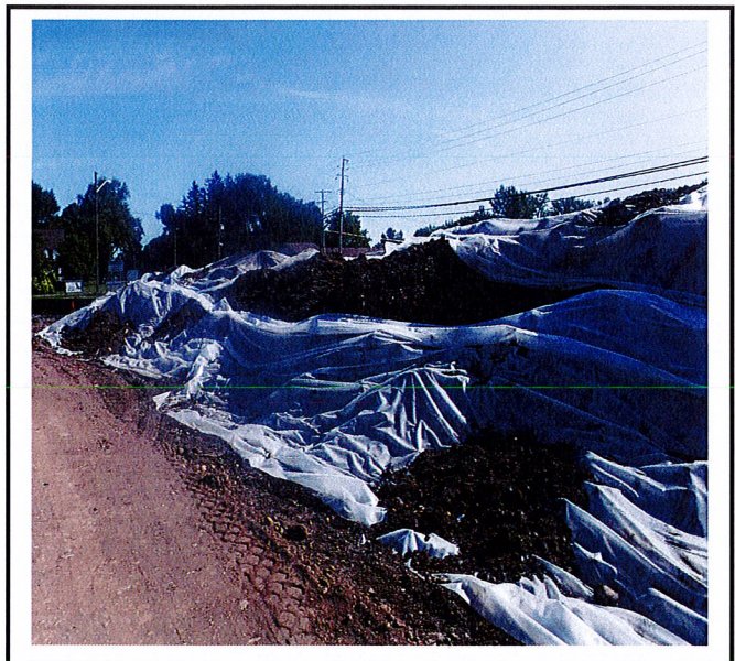
Soil stockpile is partially covered with plastic. It either has to be completely covered or temporarily stabilized.
