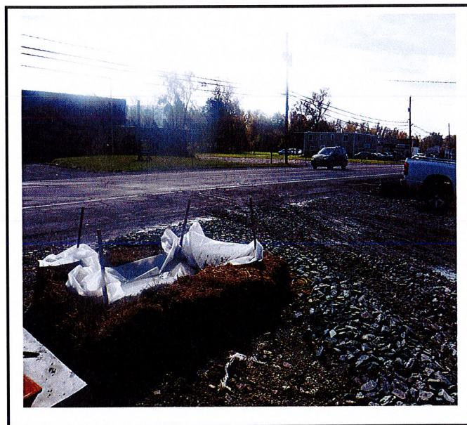
Slight mud tracking onto Old Ithaca Road. If more mud gets trucked out the road will need to be swept.
