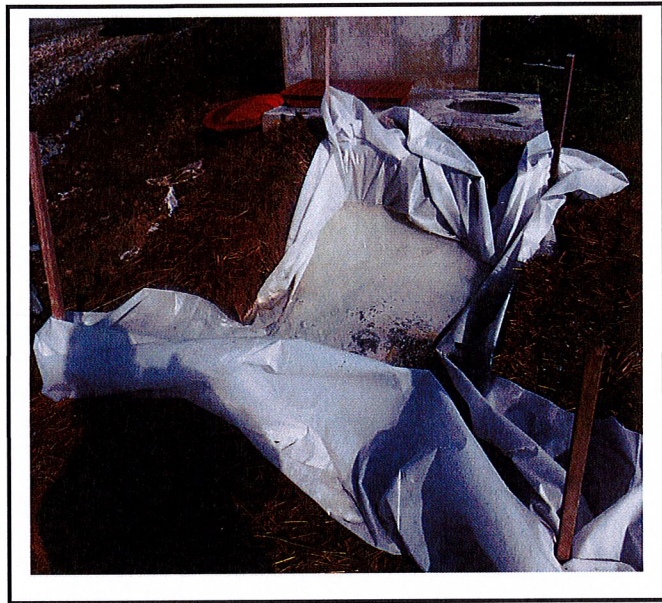
Concrete washout is at capacity and requires replacement if more concrete will be poured.
