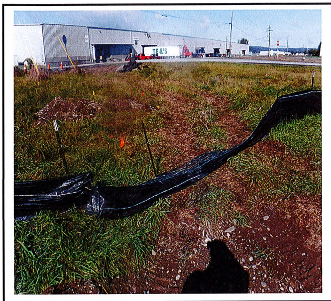
Silt fence taken down for utility work needs to be put back up.
