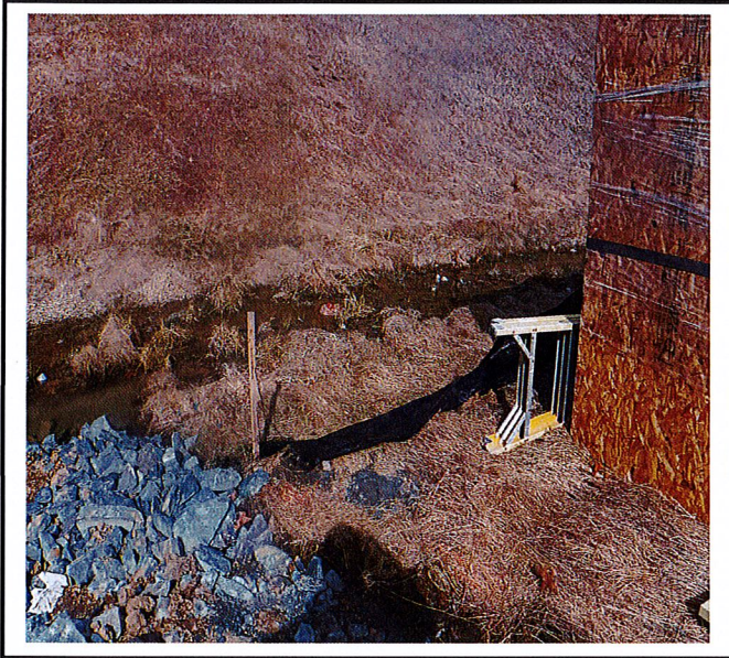
Silt fence requires repair.
