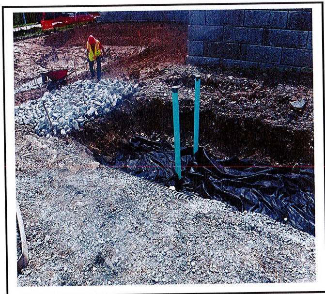
Observation ports in the south west bioretention.
