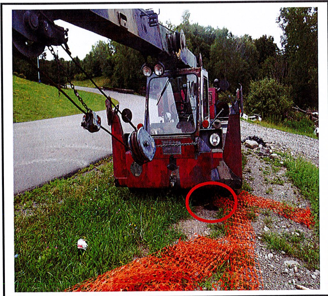
Leaking equipment is parked within the municipal ditch.
