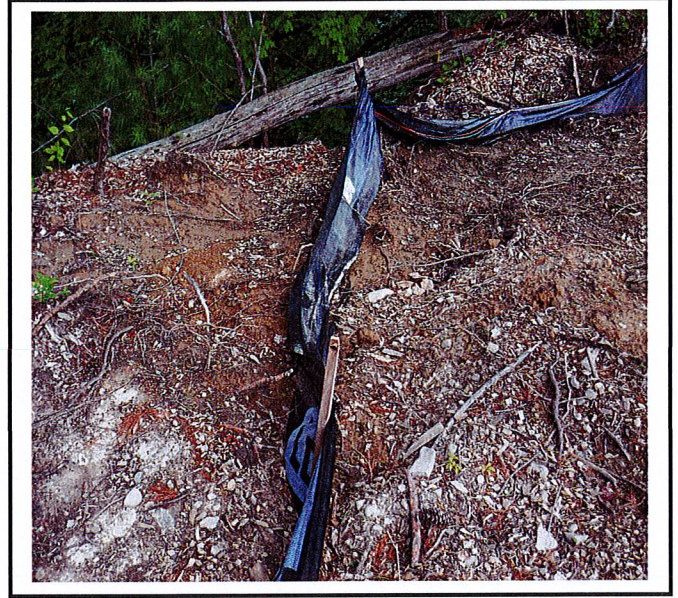
Evidence of water going over the silt fence.
