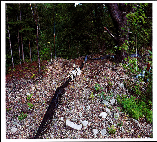
Silt fence needs to be repaired in many spots.
