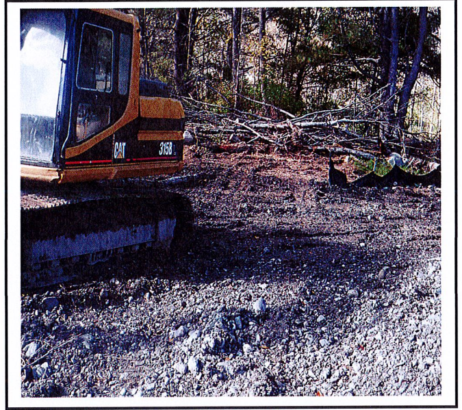
Areas have been graded where sediment controls have not been installed.
