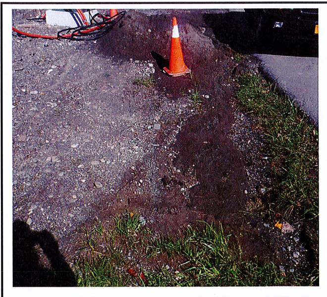
Sediment being washed to municipal ditch.
