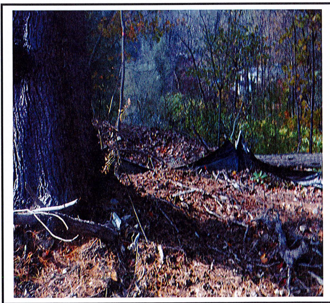
Silt fence has still not been repaired.
