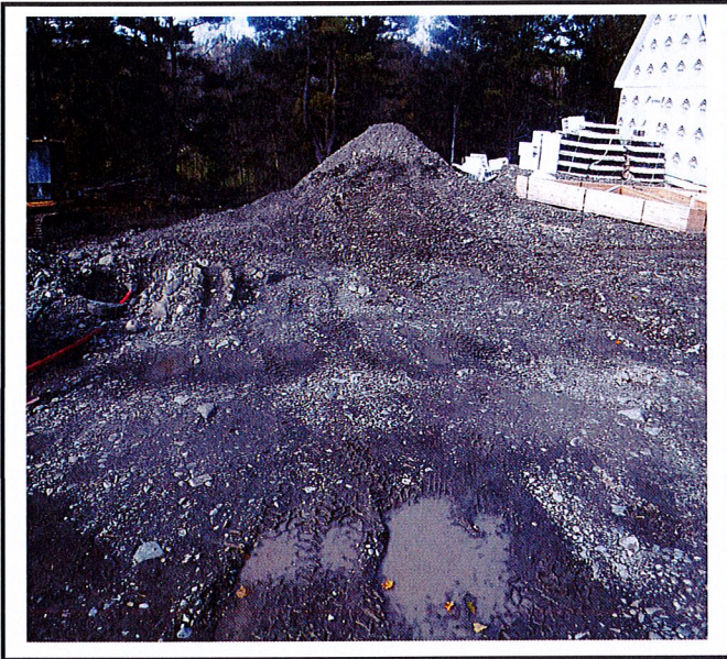
Construction entrance no longer exists.
