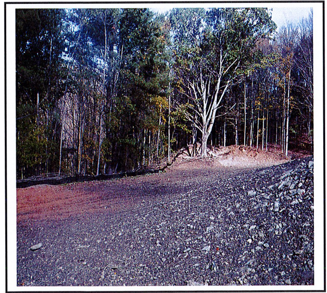
Open soils have been idle for many months with no stabilization.
