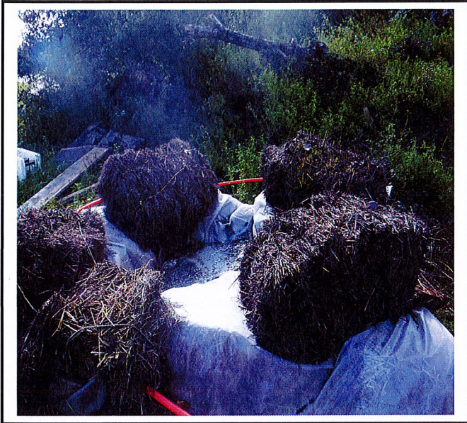
Concrete washout well over capacity. Garages are still being formed.
