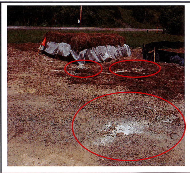
Concrete washout is installed however trucks are washing off on the ground right next to it.
