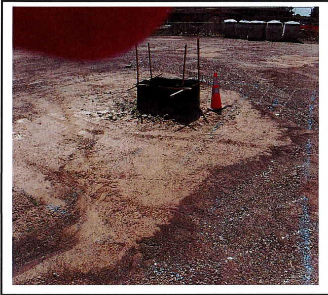
Drop inlet protection has been corrected.
