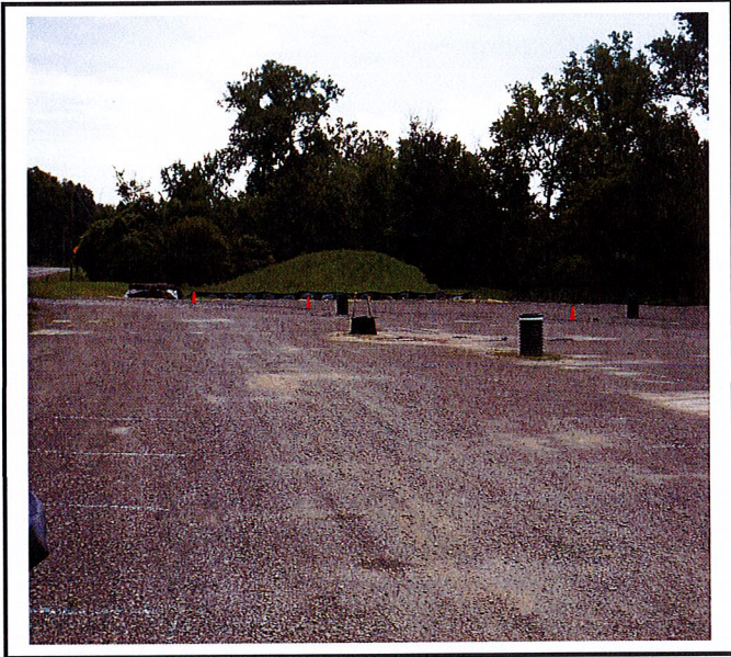
Drop Inlet structures in the parking lot and stabilized soil topsoil pile growing grass in the background.
