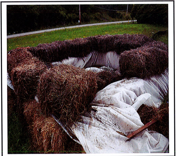
Concrete washout will need to be repaired and maintained before the next concrete pour.
