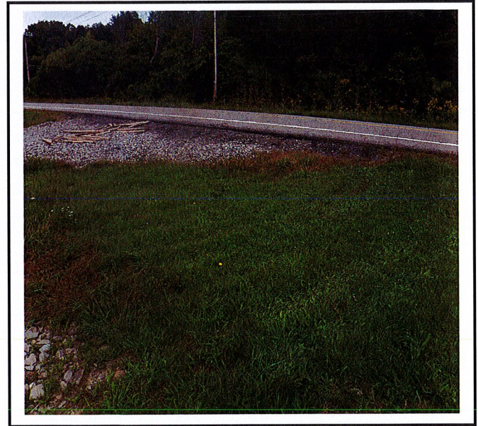
Construction entrance is being driven around because wood has been dumped in the actual construction entrance.
