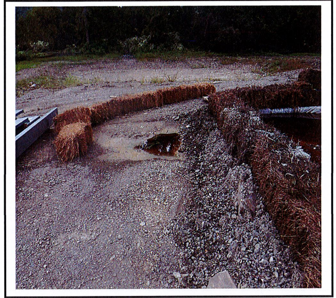
Concrete washout water has leached onto the ground.
