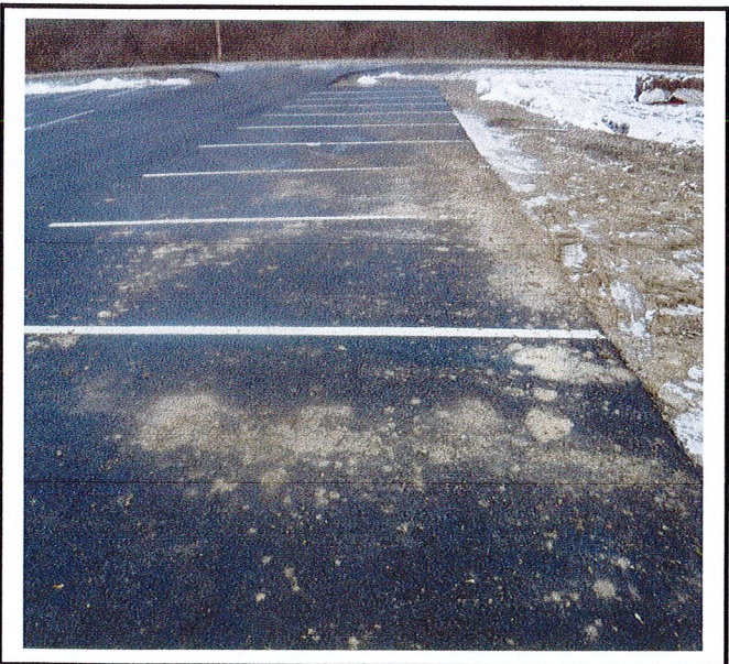
Mud is being tracked from stockpile area
