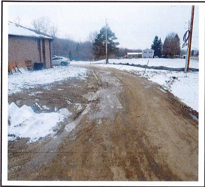
Mud is being tracked onto the old paved driveway. This mud is not part of the limits of disturbance. It is being tracked down Breesport Road.
