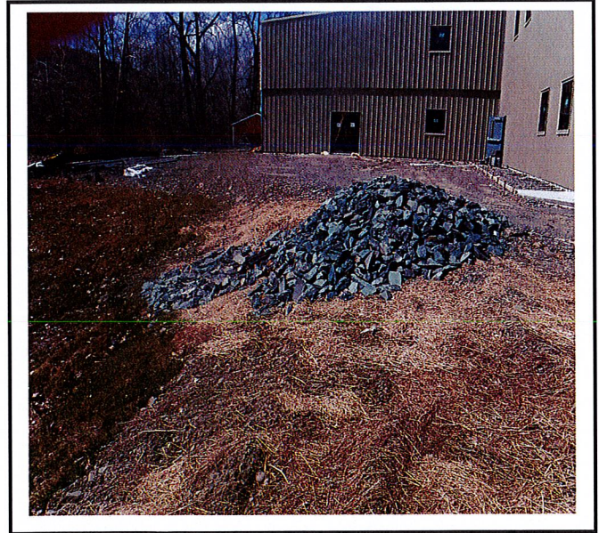
Rock outlet protections not to correct size. Rock is on site to do the work it is just not complete yet.
