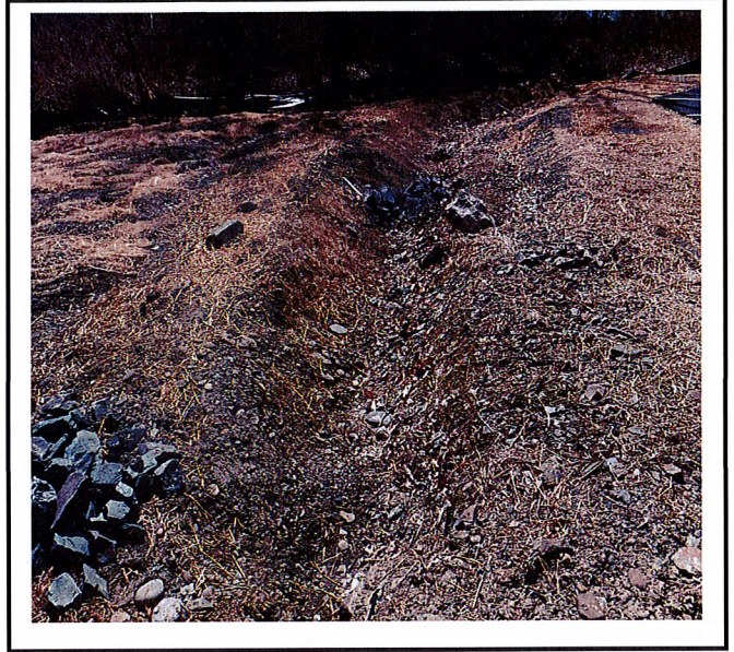
Drainage ditch to Newtown Creek- not vegetated and check dam not installed correctly.
