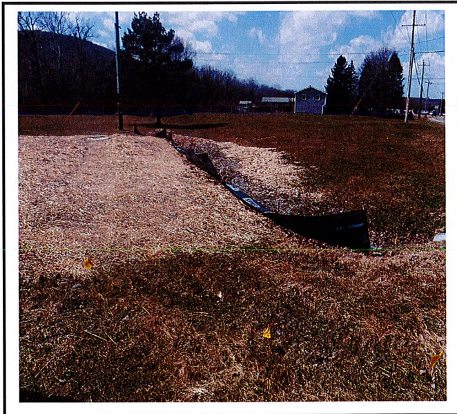
Silt fence is in need of repair and maintenance around the entire site.
