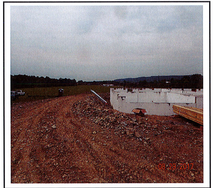
Concrete trucks are washing into basement of Building 7.
