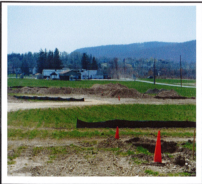
Stockpile area is being moved to this location. Once complete, this area will be temporarily stabilized.
