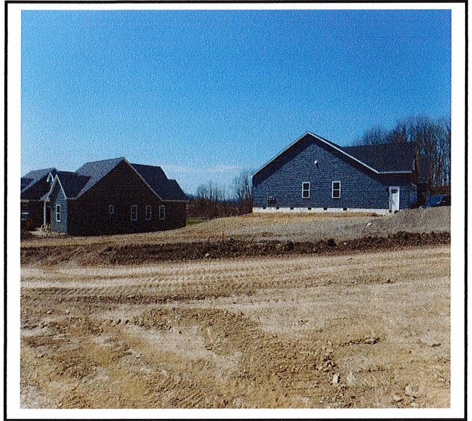
Areas around these buildings will be final grade soon and be temporarily stabilized.
