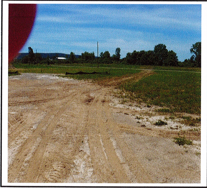
Construction entrance is not installed at the location where heavy truck traffic is entering/leaving the property.
