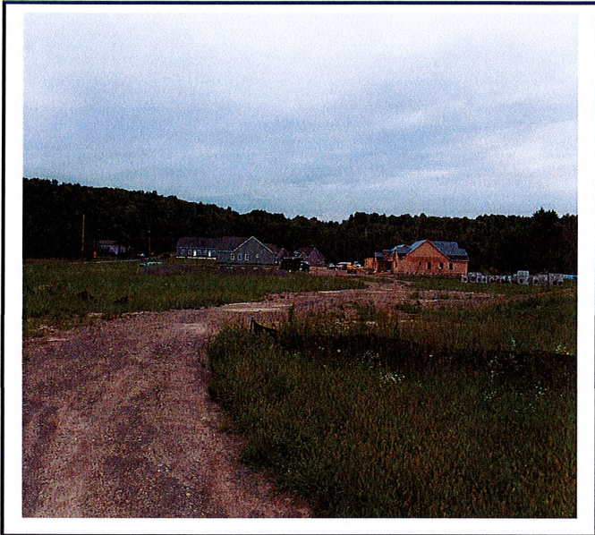
Work remains within the limits of disturbance and all idle soil has been temporarily seeded.
