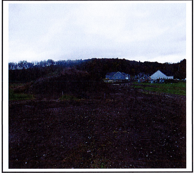
Silt fence needs to be re-installed around the soil stockpile.
