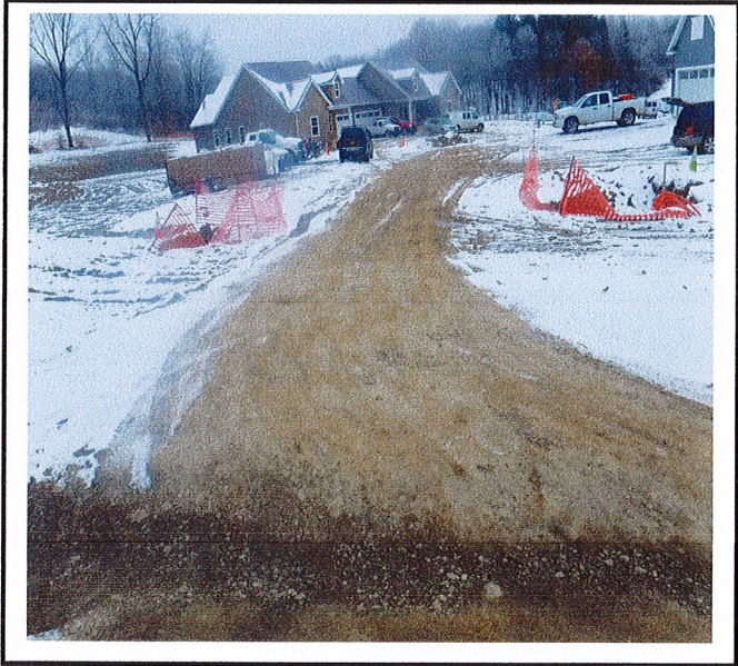
Construction entrance requires maintenance.
