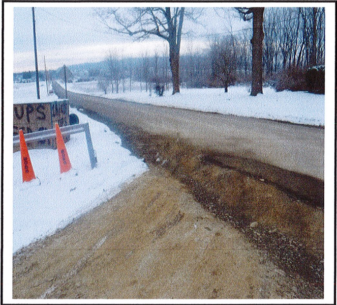
Construction entrance requires maintenance.
