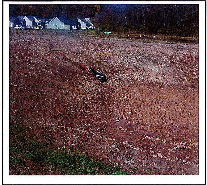
Storm sewer discharge to stormwater basin.
