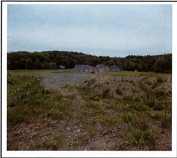
Soil stockpiles and open bare soil need to be stabilized.
