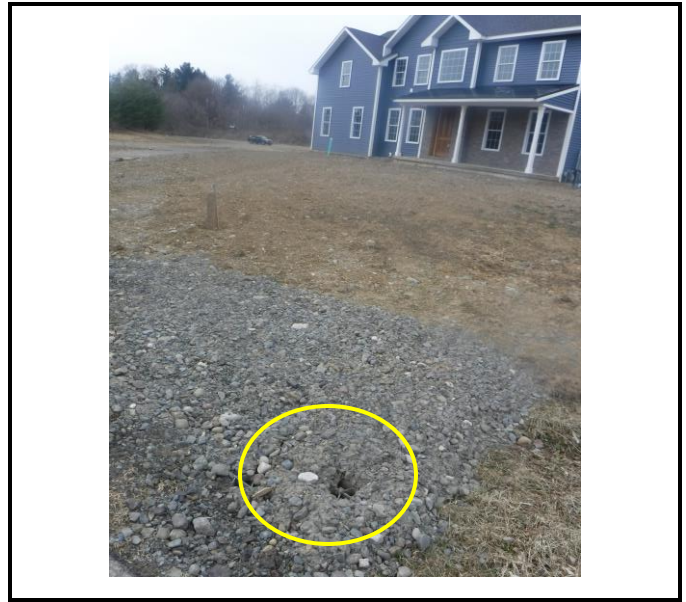
House lot that is under construction needs stabilization. The catch basin at the front of the house has been buried in stone.
