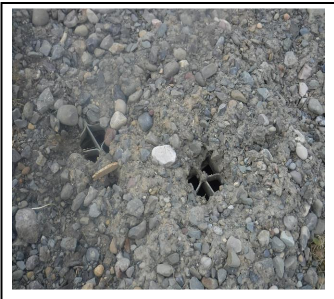
Only a small portion of this drainage structure is seen. Stone needs to be removed and proper inlet protection is to be installed.
