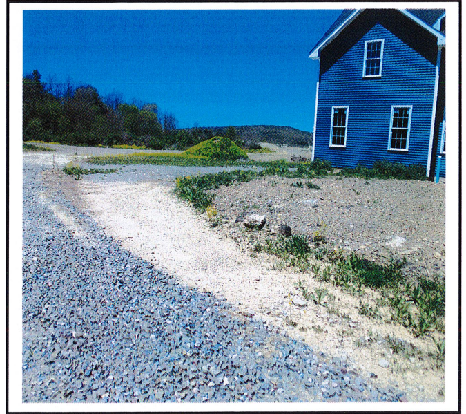
Stabilization of open exposed soil is required at this home lot.
