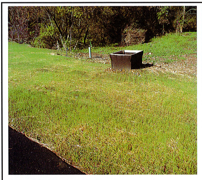
A number of stormwater structures are missing the concrete apron that directs water to drain to them.
