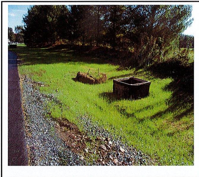
Storm sewer daylights where it should not. Straw bales in a concentrated flow is not an accepted practice.
