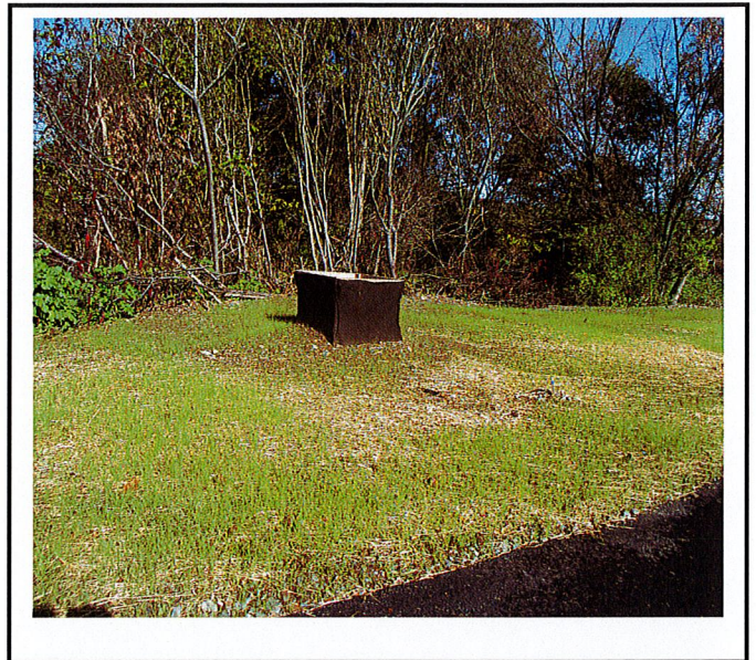
STA-10B- Structure sits so much higher than the road how will water make its way into the structure?
