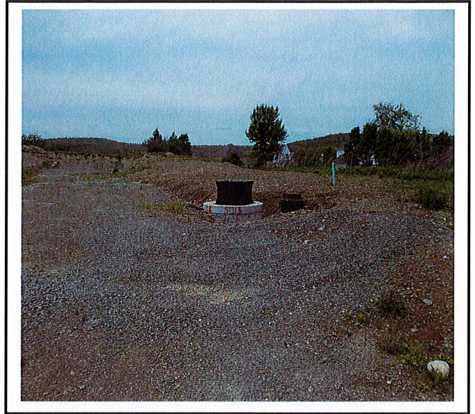
Open soil by lots 39 and 31 require stabilization.
